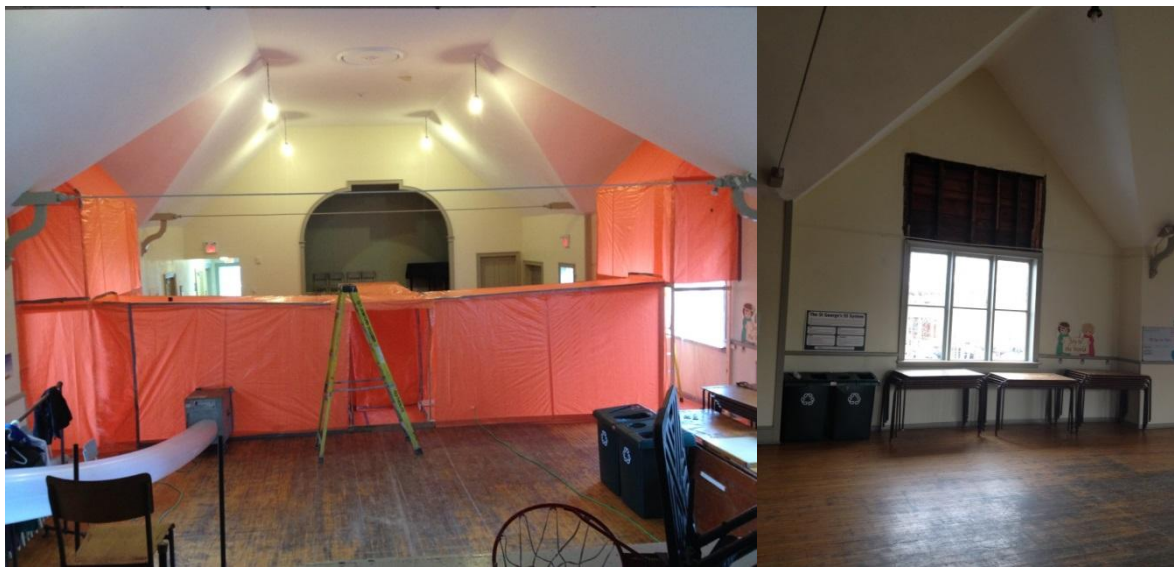
(Asbestos removal around the 2 large windows: left, for the much larger, original sizing: right)
