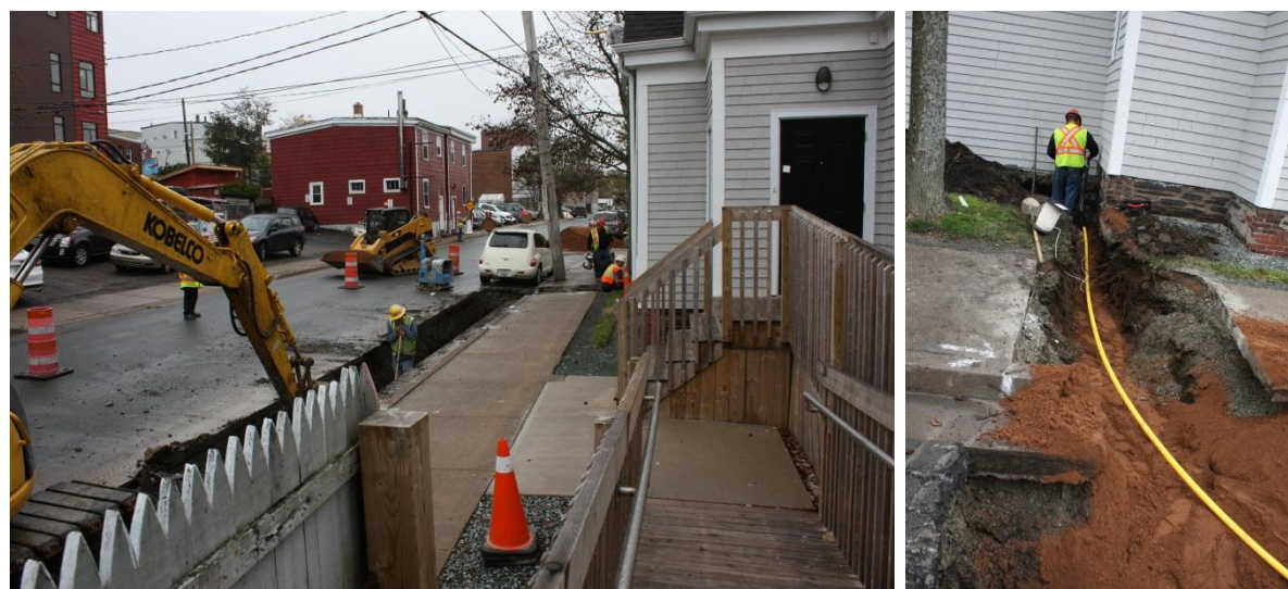
(Trenching and installation of Natural Gas to the West Side of the Hall on Maitland St.)
