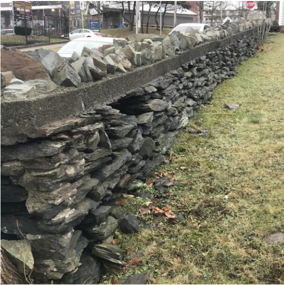
View of the wall, looking South-East towards Gerrish Street, showing missing load-bearing stones and mortar from previous attempts to repair the wall.
