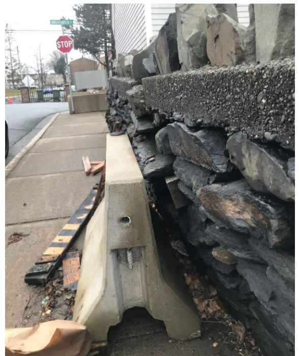
The a portion of the collapsing Gerrish Street wall, looking up the hill to Brunswick Street, showing the fractured concrete cap and the tremendous lean.
